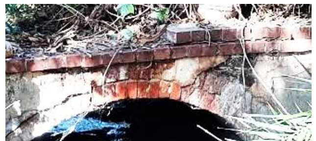
The damaged carriage bridge in the Moorcroft Court Reserve
