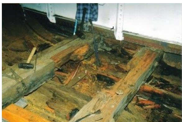
Oscar W showing deteriorated floors and keelsons before restoration
